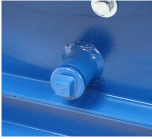
Condensate drain pipe with plug
